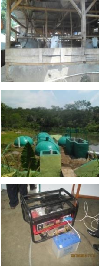
Figure 1: Biogas system in Baiturrahman Islamic Boarding School
